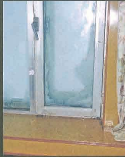
This picture shows the inside of the window in the room. Hardly surprising that a bottle of cola exploded in the cold.
